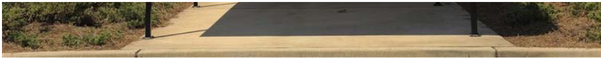
Lake Oconee Academy is expanding. A new high school facility is under construction. Terrell Clark / The Hechinger Report
